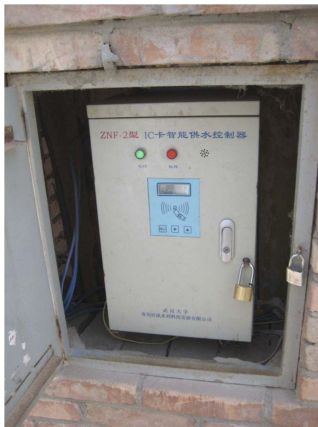
Fig. 3. The card-swipe water allocation system in Minqin County.
